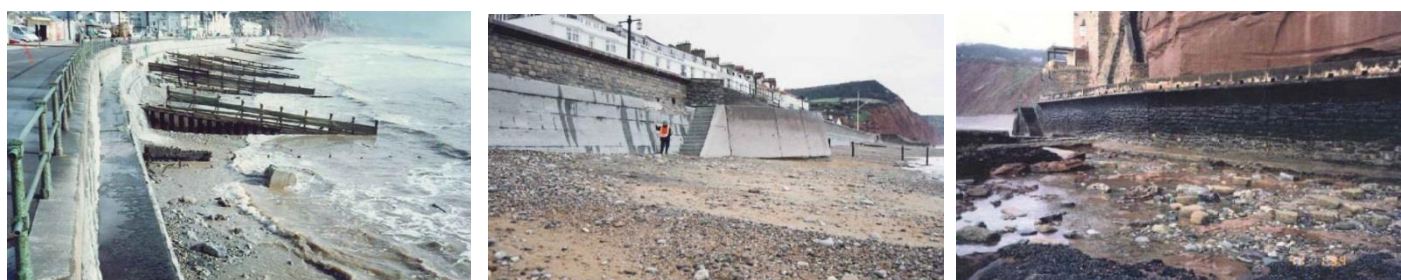
Timber groyne damage in 1990
